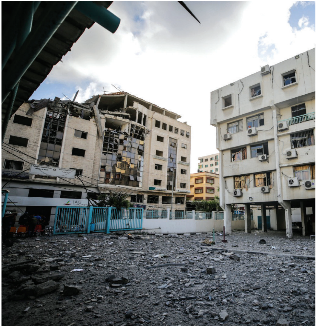
Health facilities damaged in Gaza during Israel's military offensive in May 2021. (Photo credit: Reflection Media / MAP)
