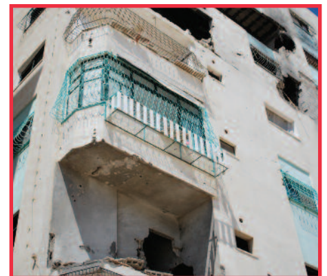
Nahlah's house suffered extensive bomb damage during the war in Gaza.
